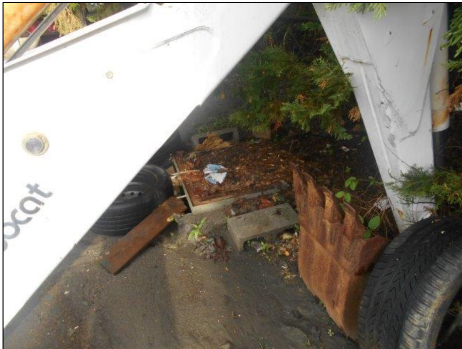
Figure 8. Open sanitary grate in the Accotink Creek floodplain
