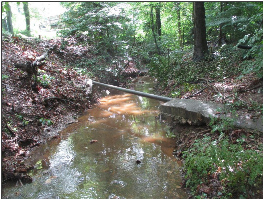
Figure 5. Erosion and undercutting of banks at the sanitary sewer crossing
